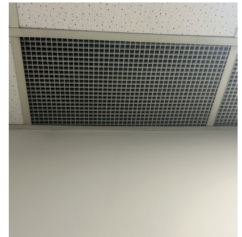
CLEAN RETURN AIR
