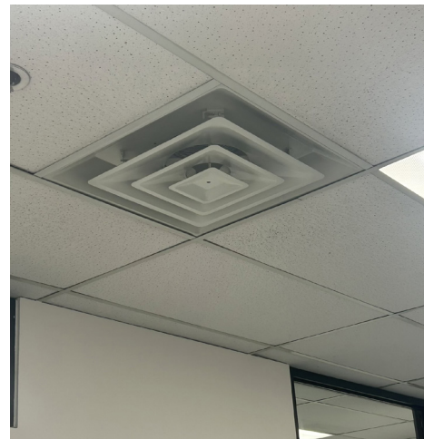
CLEAN AIR DIFFUSERS
