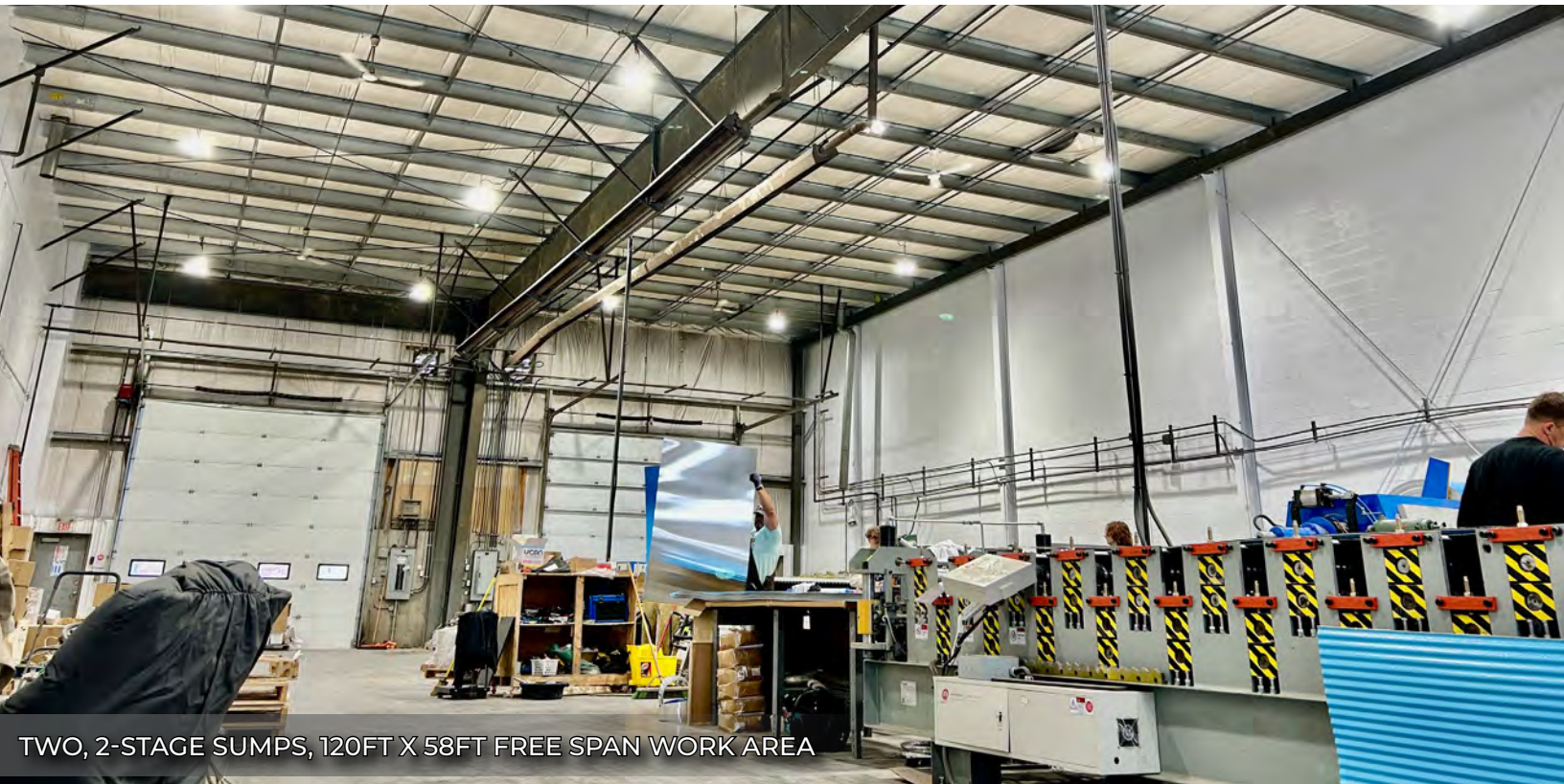
RADIANT HEAT, HIGH-BAY LED LIGHTS, FREE SPAN SHOP
