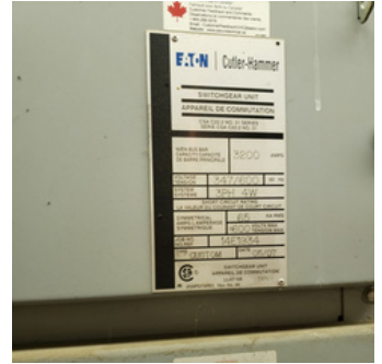
3-PHASE 3,200 AMPS / 500 VOLTS
