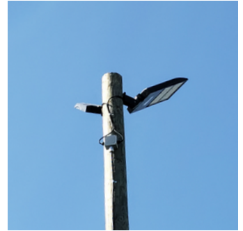
LED POLE YARD LIGHTING
